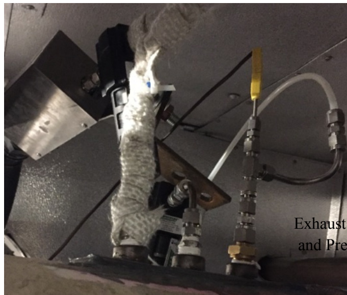
Figure 12: Back Side of Exhaust Ports on Vessel A
