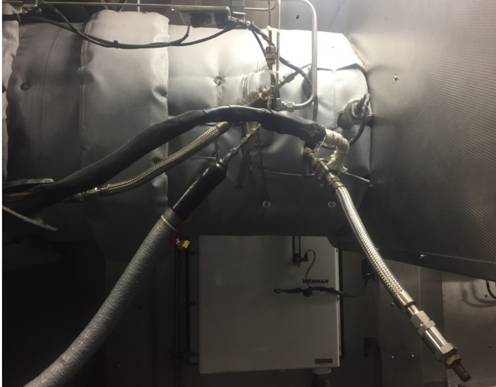
Pre-SCR sampling position in the engine room of Vessel B.
