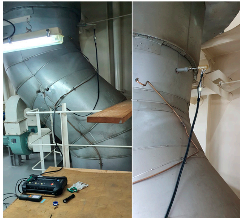
Figure 6. Position of the sampling probes during recording under real operating conditions.
